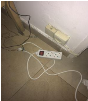
Figure 10 - Multiple electrical socket controlled by the 12V Relay
